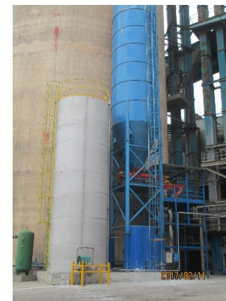
华新株洲高效水剂脱硫设施 High efficiency water desulfurization facilities on ZHUZHOU
